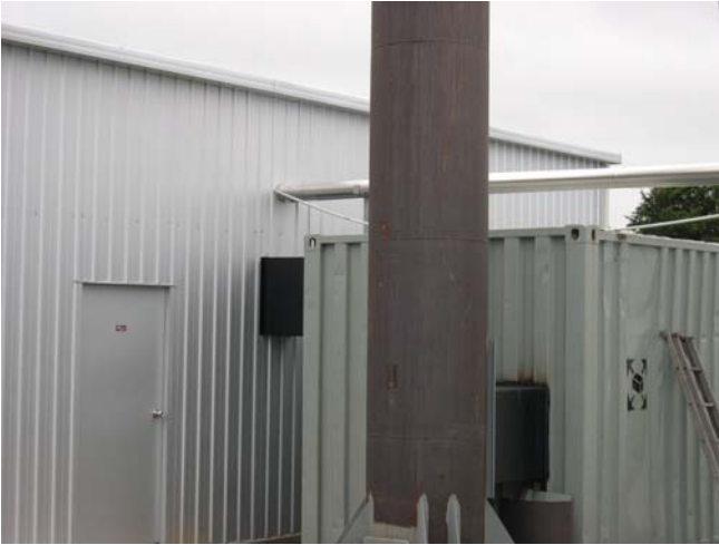
Photo 2: the latest Barton Soot Collector with connecting channels visible.
