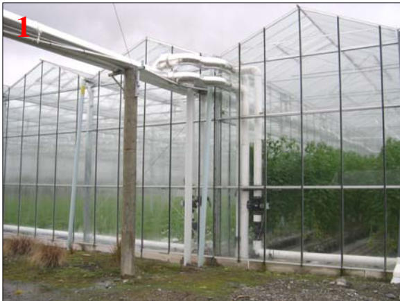
Photo 1: insulated transport pipes
