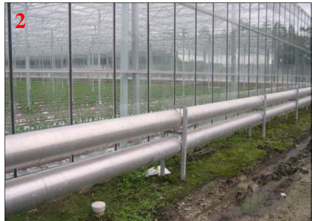
Photo 2: insulated transport pipes
