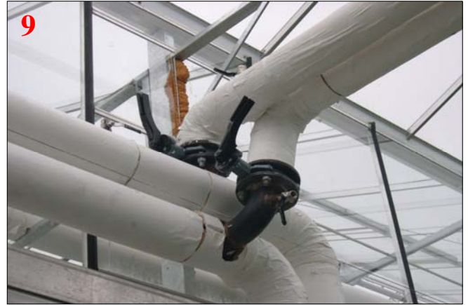
Photo 9: Example of good insulation
