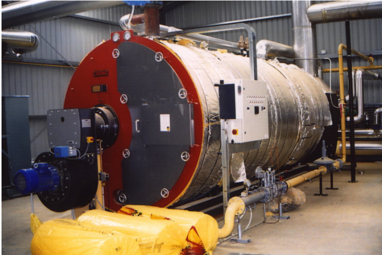
Photo 1: Most modern boilers are very efficient. Note the insulation (silver coloured). This will be covered by a stainless steel sheet.
