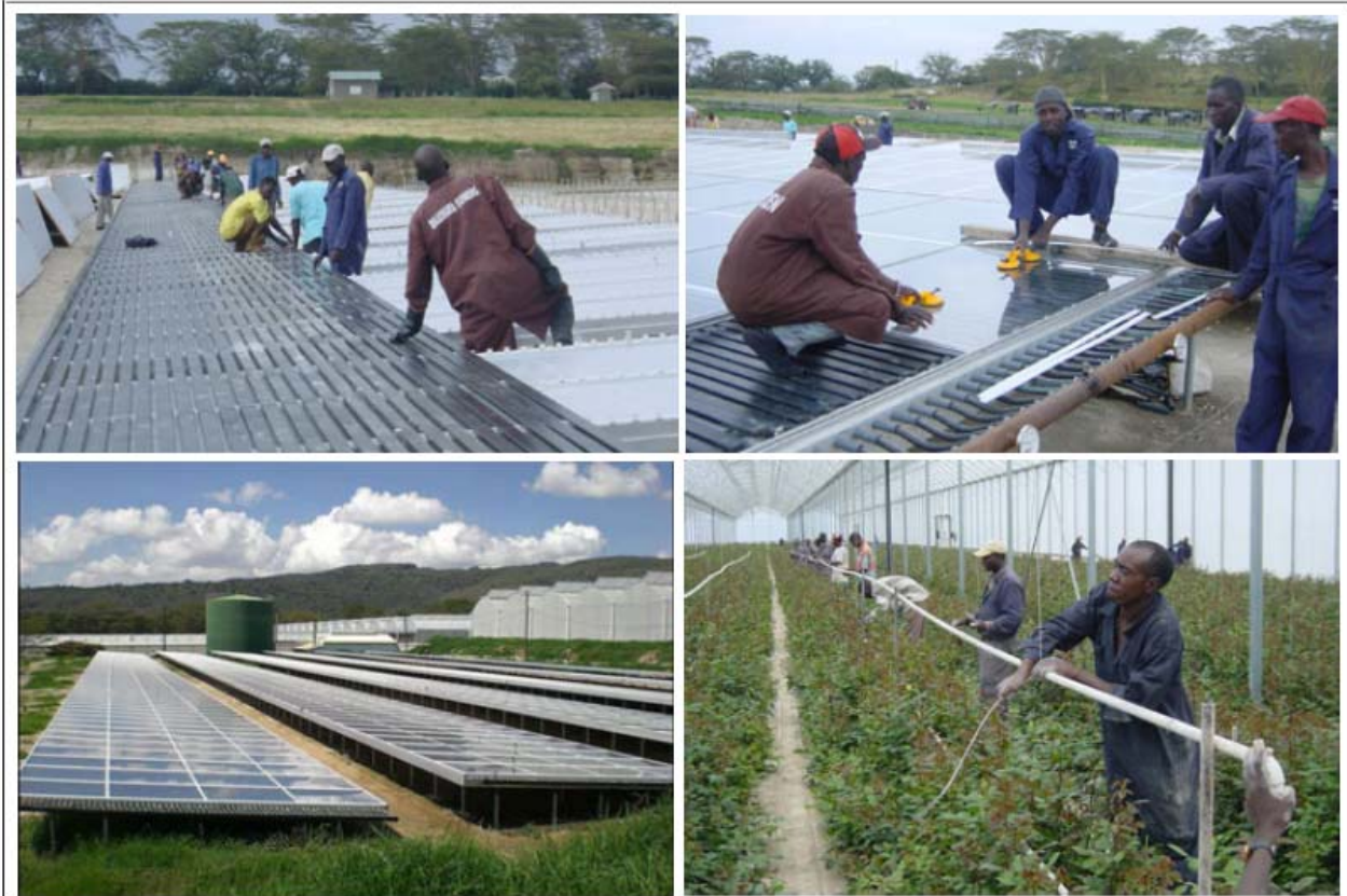
Construction of the solar collectors at Van Kleef Roses in Kenya. A total of 3,200 m 2 collectors supply heat to a 3 ha greenhouse. Black plastic rectangular 'tubes' are placed on a structure and covered by greenhouse frames and glass. Hot water pipe heating distributes the heat in the morning. Photos with permission www.vakbladvoordebloemisterij.nl .
